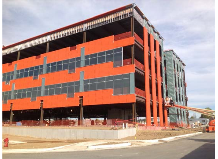
Approximately 20,000 sq.ft. of WrapShield SA Self-Adhered Water Resistive Vapor Permeable Air Barrier Sheet was installed.
