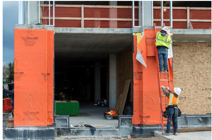
Over 100,000 sq.ft. of WrapShield SA Self-Adhered is being installed on the Hyatt Regency Hotel in Seattle, WA.
