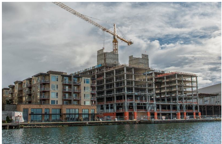
WrapShield SA Self-Adhered was chosen for its ability to be applied in the windy, wet weather conditions of Washington.
